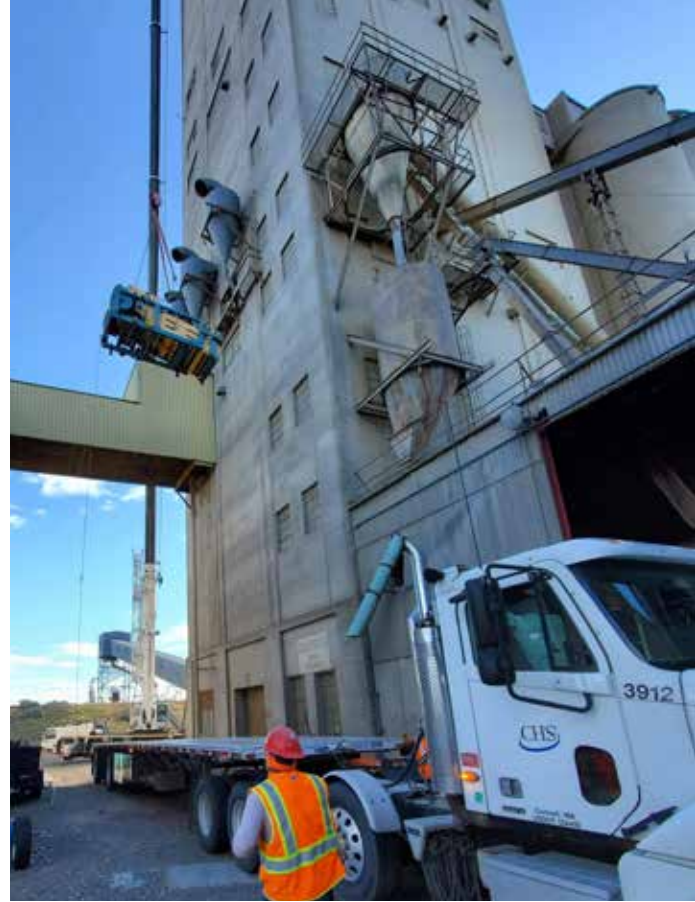
The Kennewick facility is receiving a $5.6 million upgrade.
